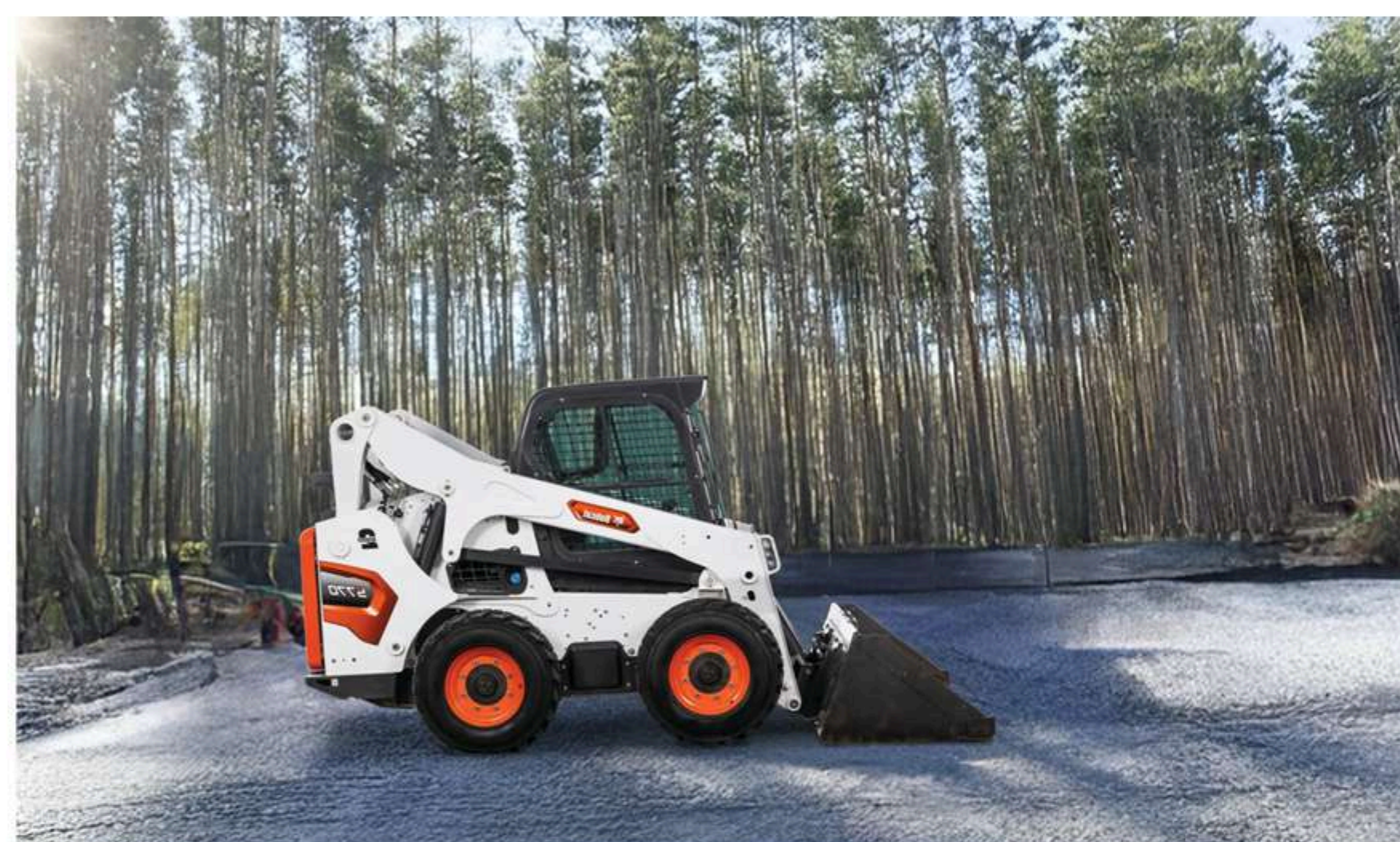
Figure 28 - Utilizing a skid steer (ideally with a spreader bar) to efficiently infill TREX.
