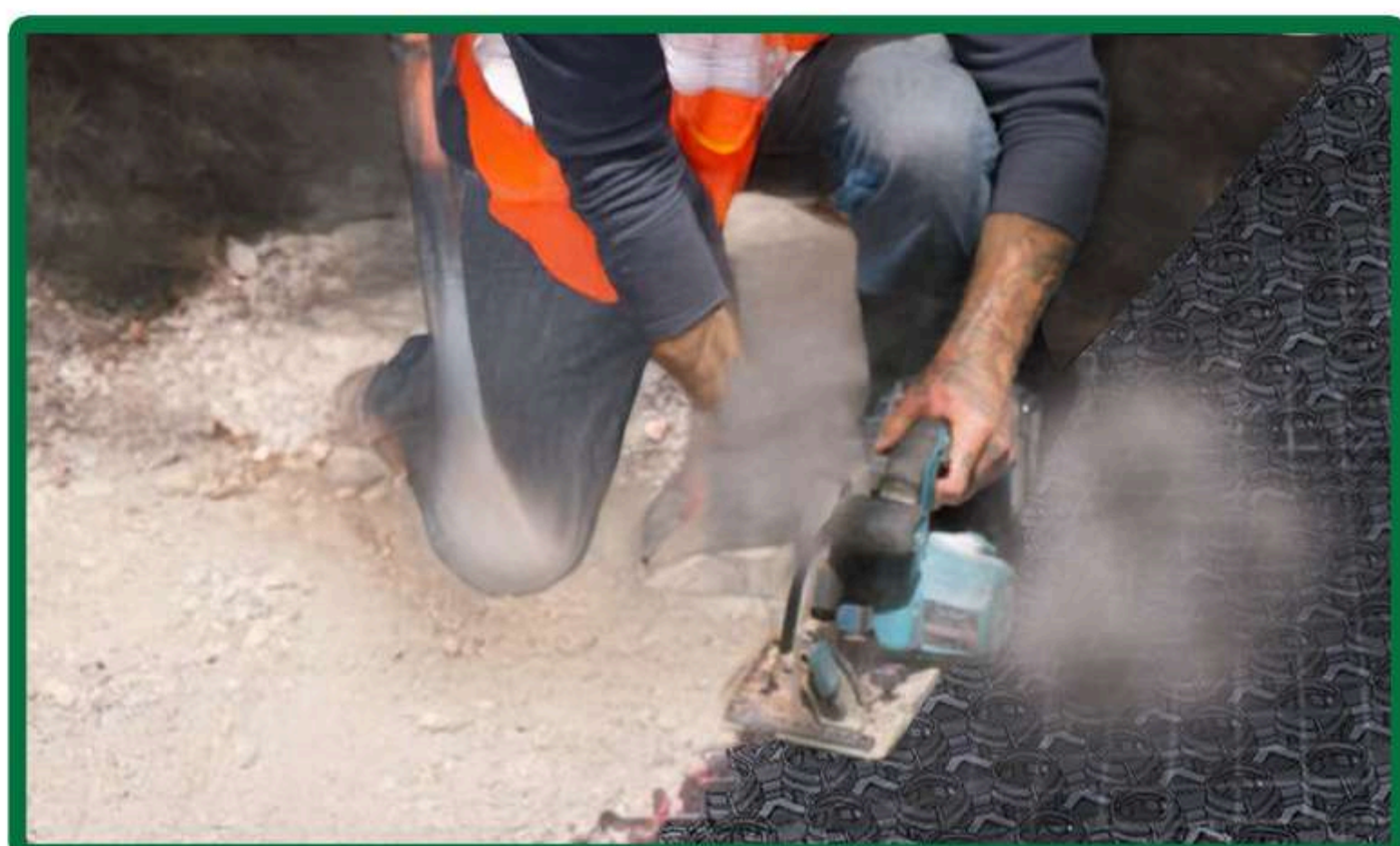
Figure 26 - TREX cut and ready for fill. Offcuts can be used on the opposite side ensuring minimum wastage.
