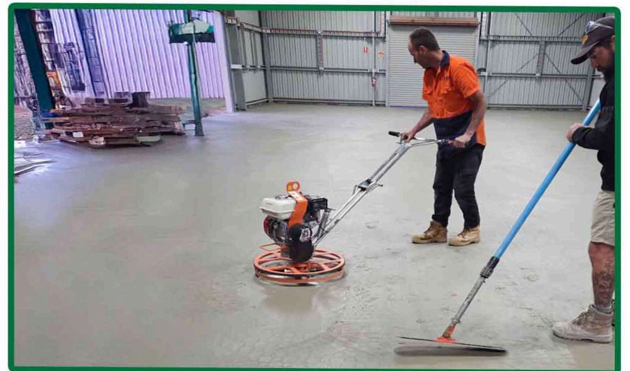
Figure 13 - Spread concrete evenly over TREXLOK, filling all spaces by hand with rakes and squeegees or vibrating screed for larger projects.
